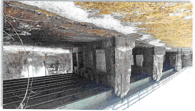
Figure 24 Looking north at the Route 9H bridge. The AHET will pass under the bridge opening on the right side of this picture
