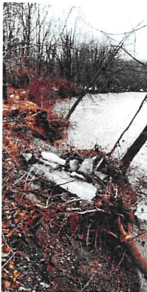
Figure 4 Eroding shoreline at the River Street Park
